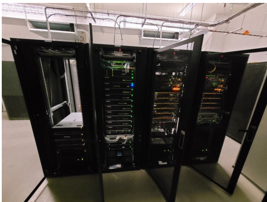
Figure 4.6: Bucharest Data Center
